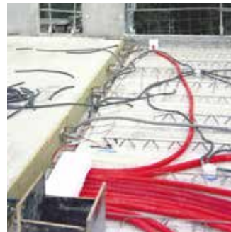
❷ Phase 1 concreting and Phase 2 Titan dowel positioning. The springs are positioned.
